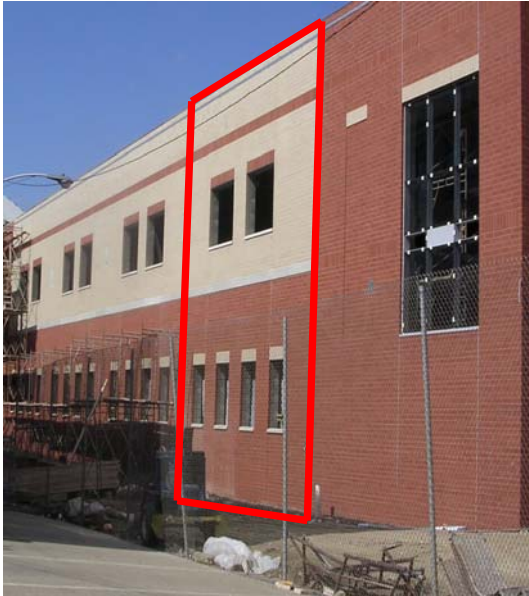
Conventional brick and CMU façade as built with area of precast panel outlined.
